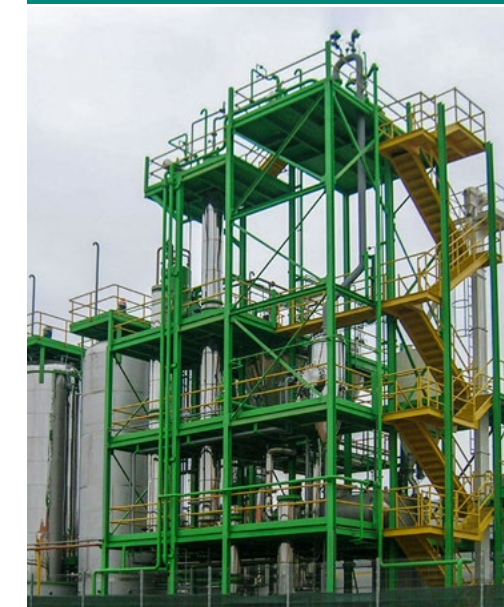
PERSEO Bioethanol® Pilot Plant
